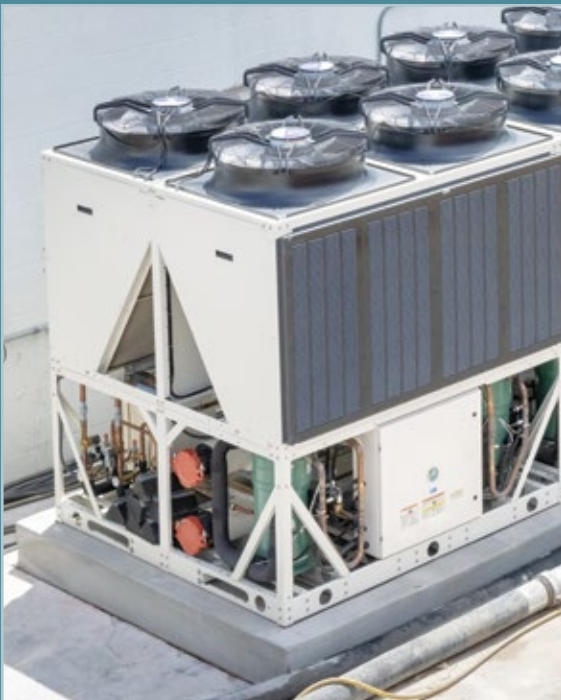
Dry-cooled evaporative cooling system
