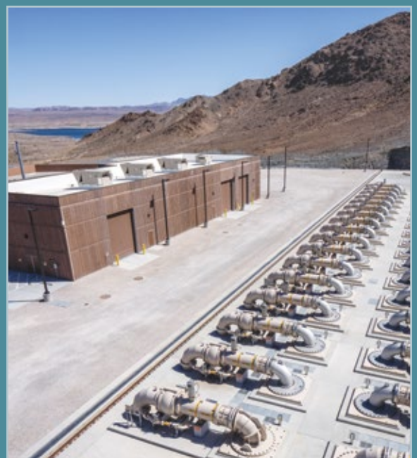
Low Lake Level Pumping Station
